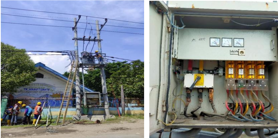
Figure 1. Transformator 160 kVA PT. PLN ULP Kenjeran
