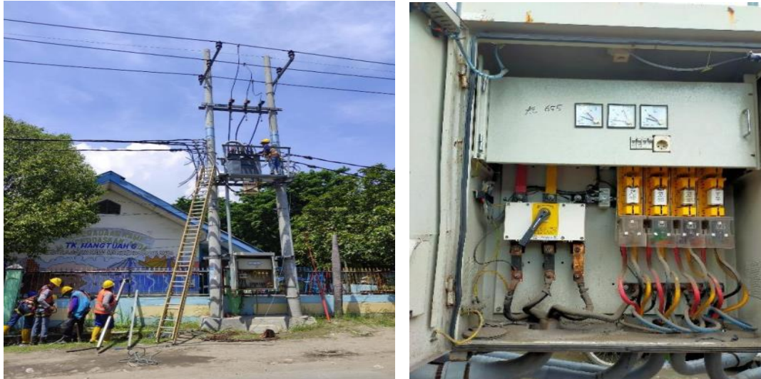
Figure 1. Transformator 160 kVA PT. PLN ULP Kenjeran
